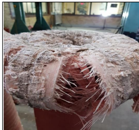
Figure 2. Localised failure at the end of the pipe stick, showing breakage of circumferential fibres
