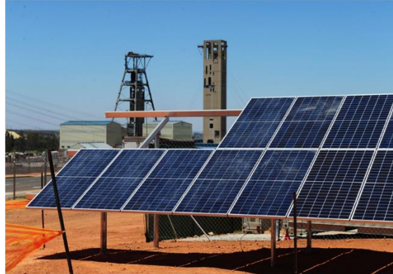
Figure 32: Gold Fields' Solar Plant
