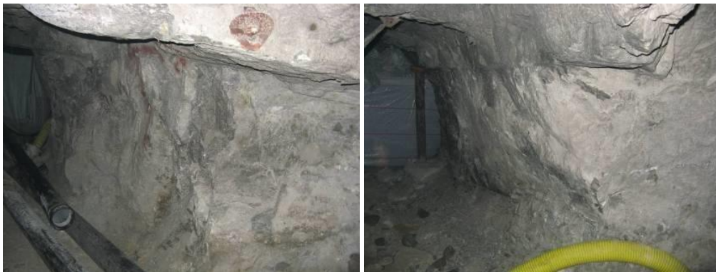
Figure 11. View of the other edges of pillar A. Less spalling was seen on these sides of the pillar
