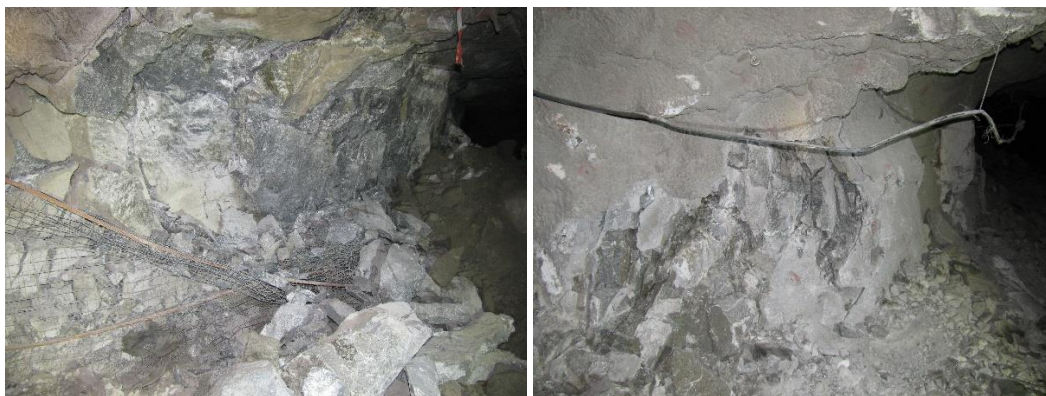
Figure 55. Examples where the pillar support failed. This is some distance away from Area A
