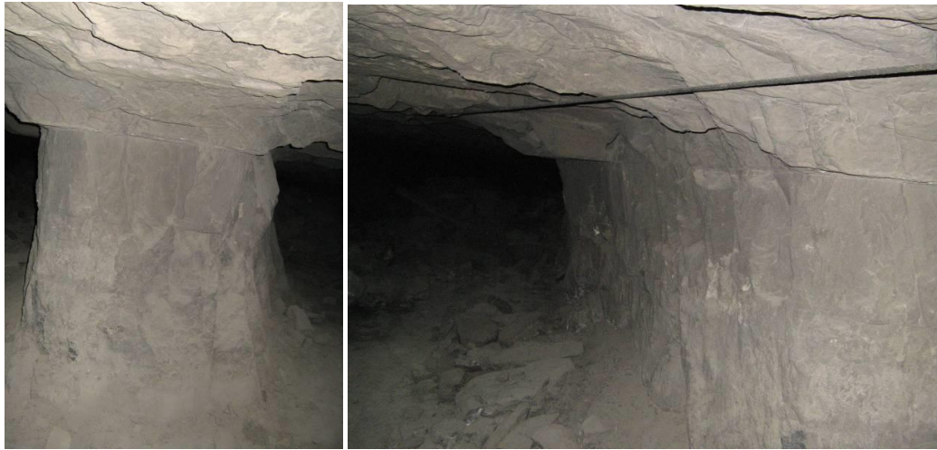
Figure 44. Condition of pillar P227
