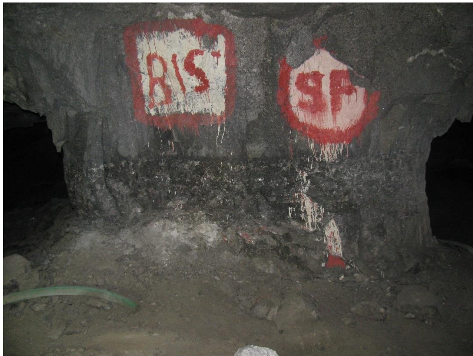
Figure 69. Another photograph of the typical condition of the pillars in the N1E and N2E areas of Styldrift Mine simulated in 2021. The joints appear to be less prominent than shown in Figures 66 and 67
