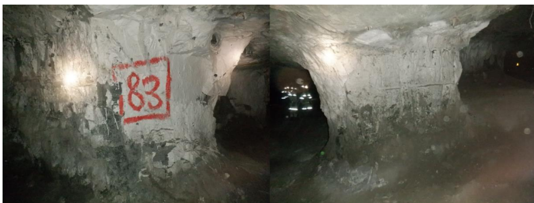
Figure 86. Photographs illustrating the condition of S75 DD P83
