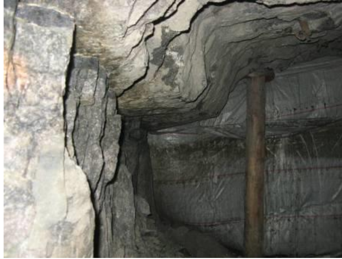
Figure 24. Signs of possible time-dependent spalling. Note the original position of the edge of the pillar and by how much the anorthosite and chrome stringer has scaled out
