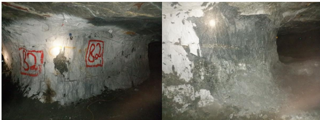
Figure 85. Photographs illustrating the condition of pillar S75 DD P82
