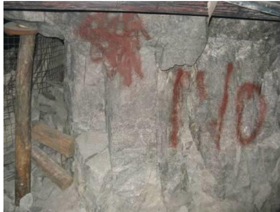
Figure 13. View of one of the corners of pillar B. Some spalling could be seen in this corner and it appears to be caused by the opening of pre-existing joints
