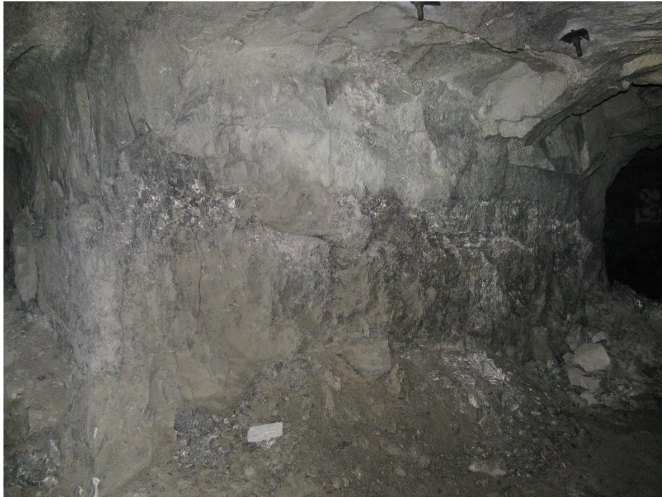
Figure 68. Typical condition of the pillars in the N1E and N2E areas of Styldrift Mine simulated in 2021. The joints appear to be less prominent than shown in Figures 66 and 67
