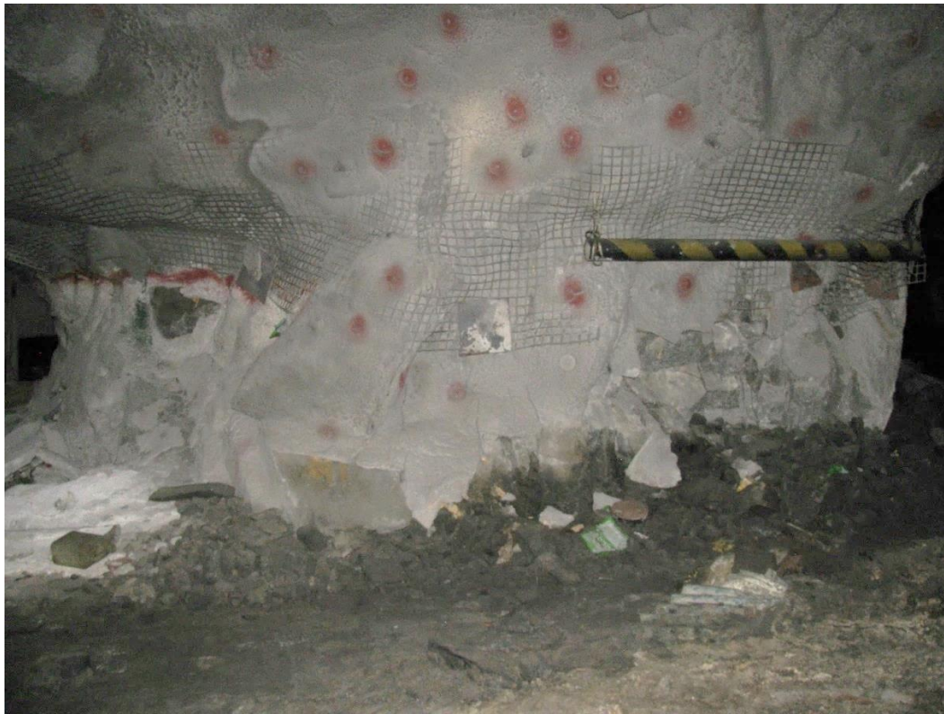
Figure 54. Typical condition of the older pillars in vicinity to Area A
