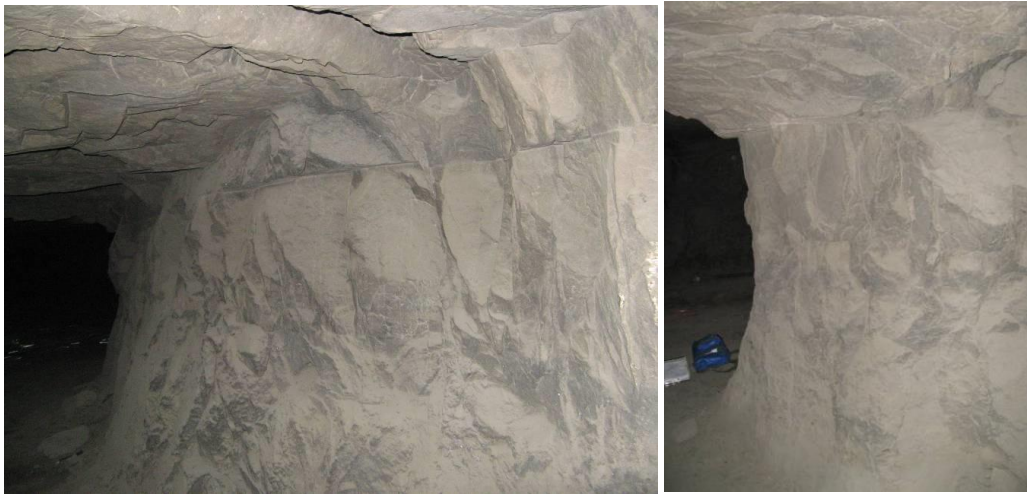
Figure 45. Condition of pillar P227
