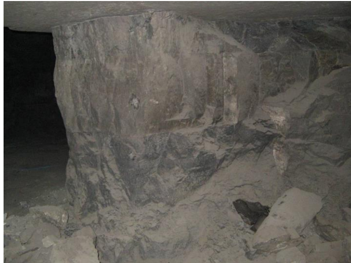
Figure 47. Condition of pillar P241
