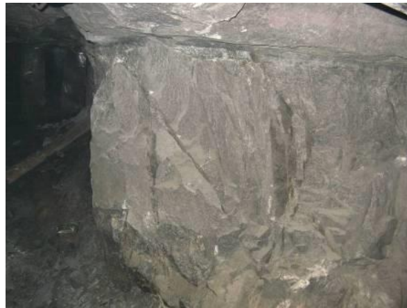
Figure 14. View of one of the corners of pillar C. Some minor spalling could be seen on this corner
