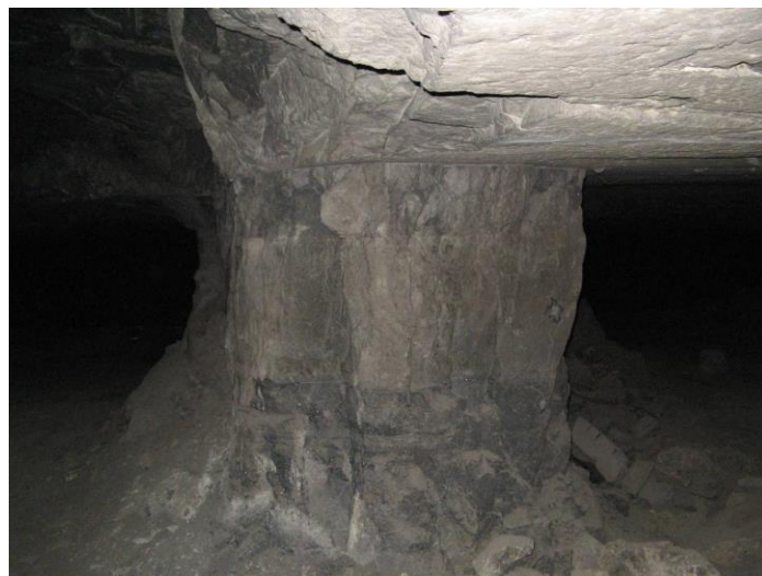
Figure 46. Condition of pillar P241
