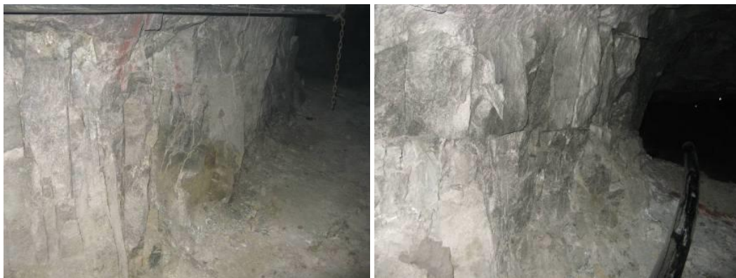
Figure 12. Views of the sides of pillar B. Less spalling was seen on this pillar compared to pillar A
