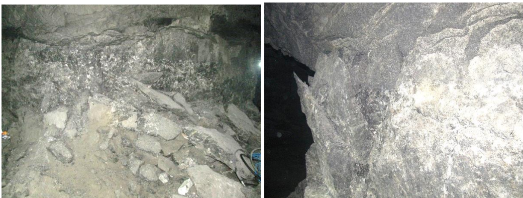
Figure 5. Extensive spalling seen for some of the pillars in Section N1E
