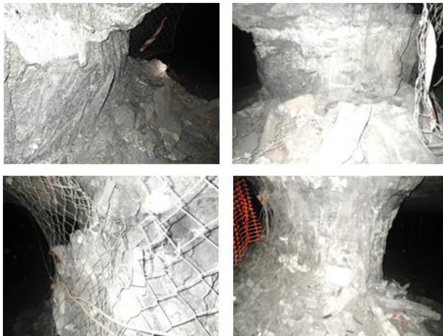
Figure 30. A “Class 5” failed pillar in the pillar project area
